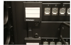
Labeling system mounted
