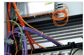
Fiber optic and copper cabling in media broadcast vans
