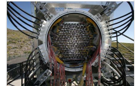
Fiber optic cabling of detector
